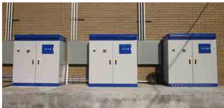
Carlstadt, NJ - USA, 300kW: KACO XP100U, 2011
